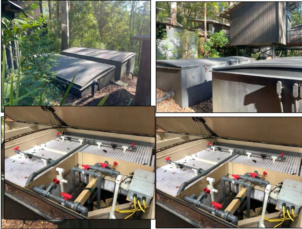
Image 1: Dual AX-Max Units installed at the Woodcutters EcoCamp
